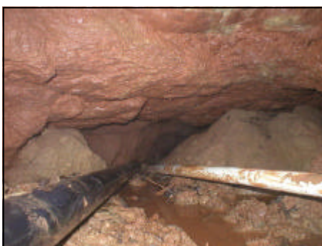
The water disposal system
