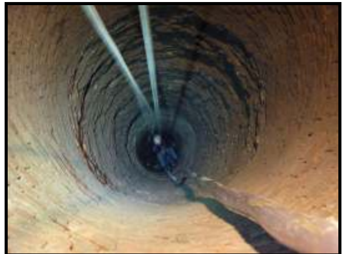
Paul near the bottom of the well. Note the brick lining. Photo: "Biff" Frith
