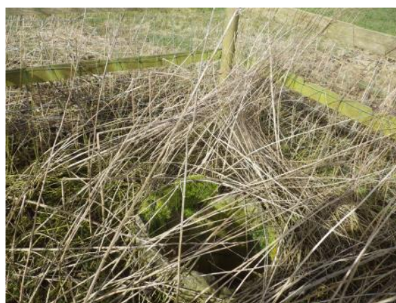
Close up of pipe Photo by Mike Moxon
